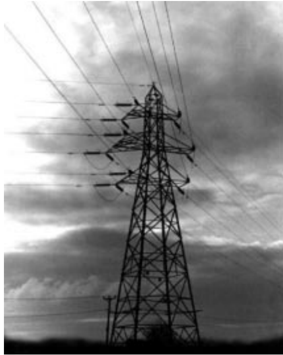
Fig. 10: Trellis mast for high-voltage cables.
